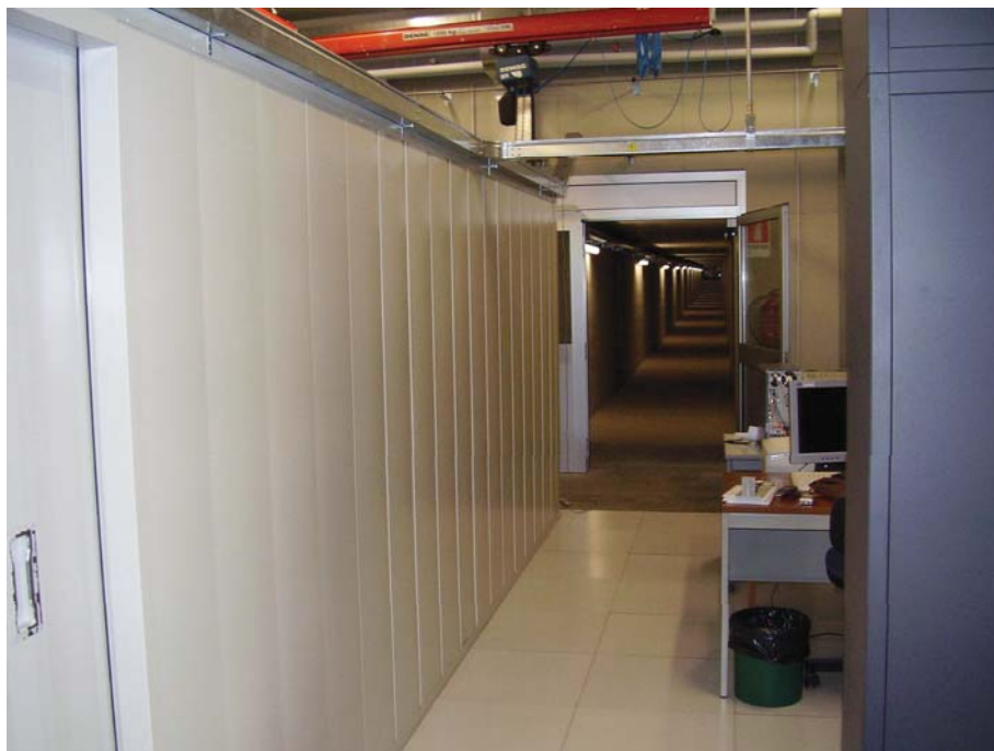
The LARIX A facility and The Console Room
